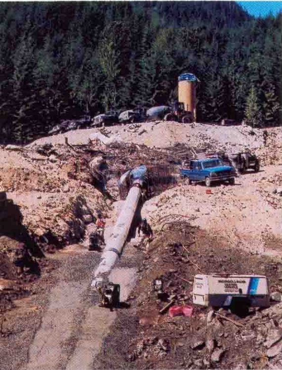
Compacting fill around the exposed pipe on a 67% grade posed many challenges.
