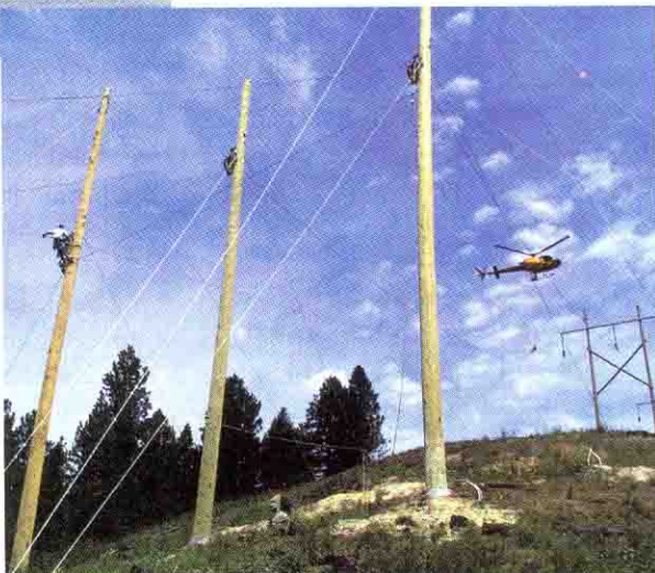
Flying over uneven terrain often makes the job of stringing conductors very tricky.
