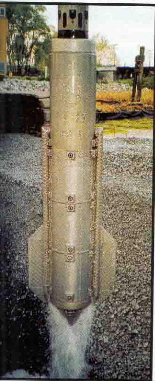
A vibrofloat probe was used to build stone columns to strengthen soil mass under bridge.
