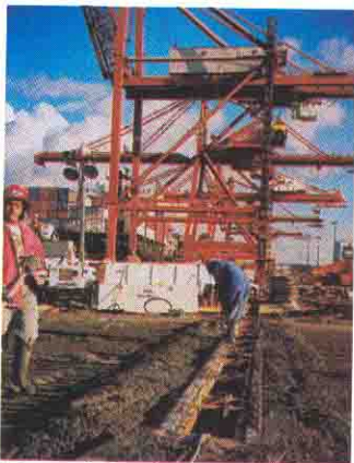
One of the job's more challenging aspects was building the extended gantry rails designed to handle massive loads
