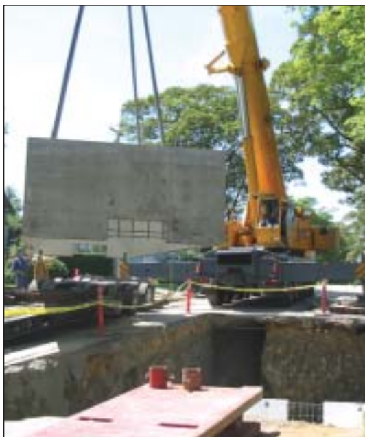
Top: The exit pit shows the completed tunnel with all carrier pipes. A grout tube is also shown. Bottom: Massive concrete manhole/vault being lowered into the ground.
