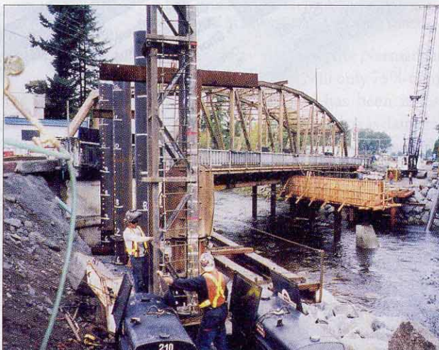
▲ Changeover. Two-lane steel bridge will give way to four-lane segmental concrete model.
