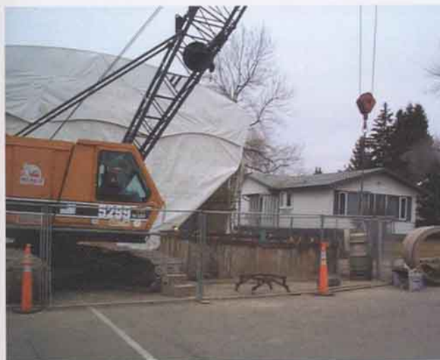
Left: Proximity of the working shaft to the neighbors with the operating equipment protected from the cold in the erected tent
