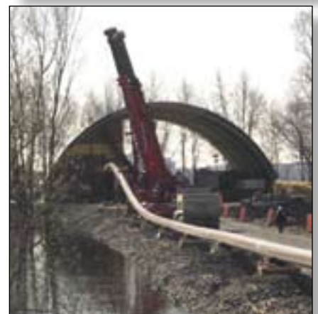
Top: One of the large downhole tools used on the project. Middle: Pipe is readied for the pullback. Bottom: The pipe string stretched beyond the shelter and dam.
