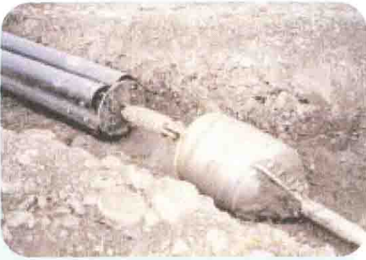
Four cables are getting ready to pull the conduit under the Fraser River from Kidd #1 substation to Mitchell Island (distribution line).
