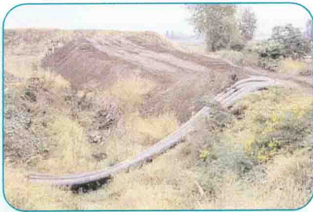
Laying out the pipe before it is pulled through the hole under the Fraser River.
